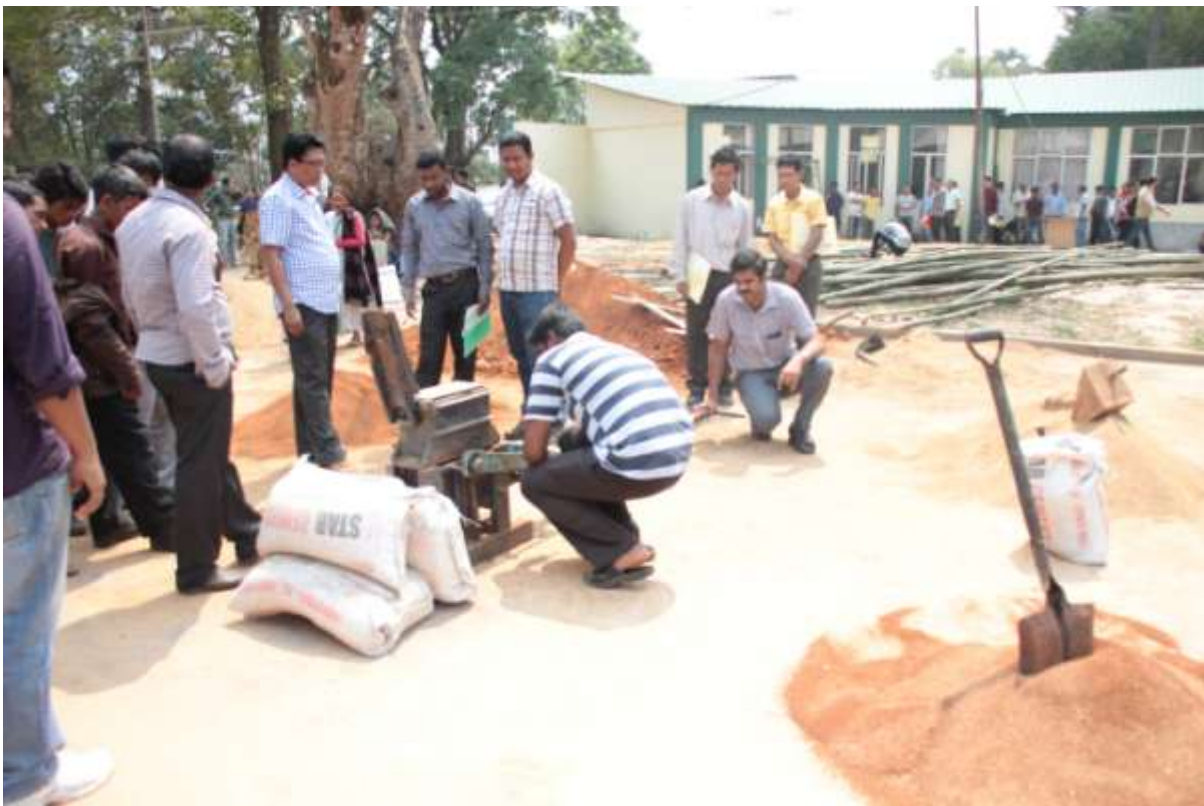
Picture 14. Making CSEB blocks using the Mardhini press. The mould is being prepared. One can see the sifted sand, and soil in the vicinity.
