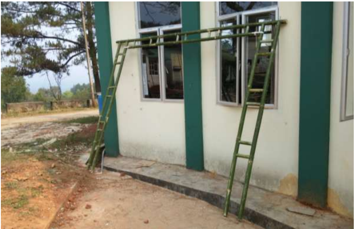
Picture 24 Bamboo columns and beam forming a portal. Small dia. Bamboos (approx 40 mm) were used for this.
