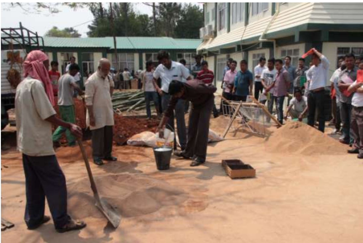
Picture 7 Mixing lime into the water that will be used in the soil and cement mix for block making.
