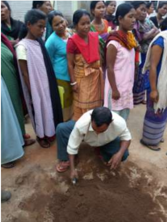
Picture 12 Mixing of the earth, sand and cement mix for CSEB and rammed earth production
